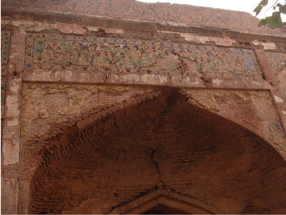
Figure 2: Perimeter wall -Decayed tile mosaic and plaster work on the gate
